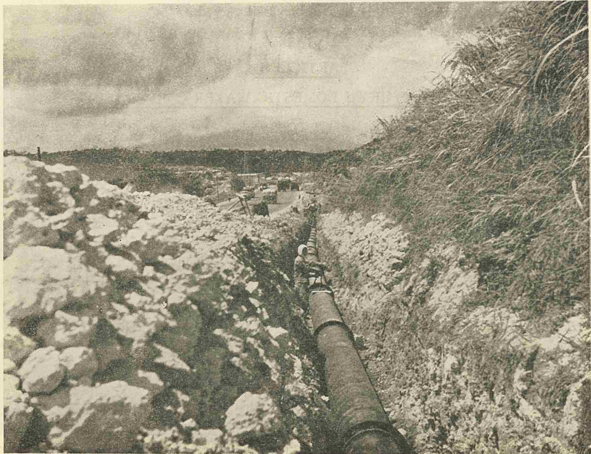
Inastallation of 16" water main on Route 1. The main runs from Kakazu Pumping Station to Naha Water Treatment Plant at Tomari
