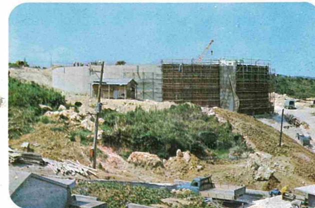
Ojana 5MG Storage Tank
