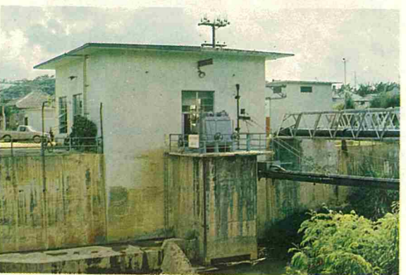
Kawasaki Pump Station
