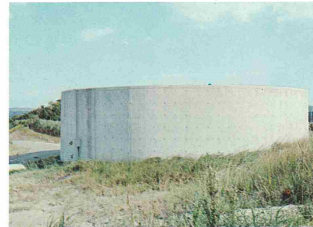
Tomigusuku Storage Tank ( 0.5 MG )
