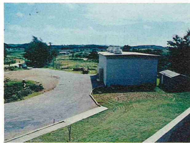
Tengan High-Lift Pump Station ( 13 MGD )
