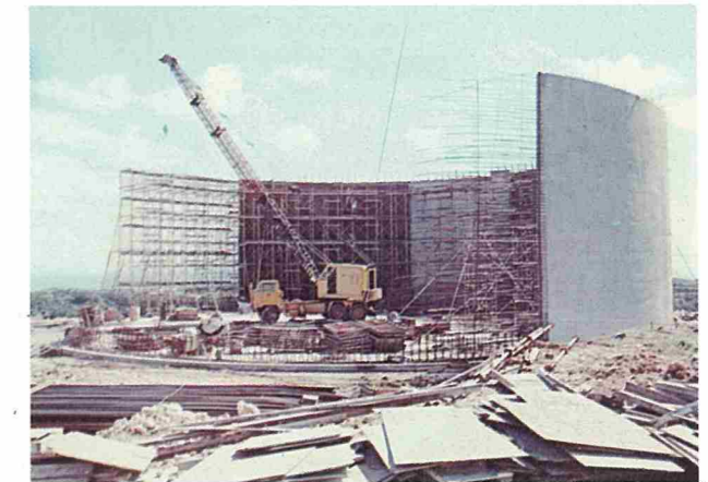
Yokatsu Storage Tank
