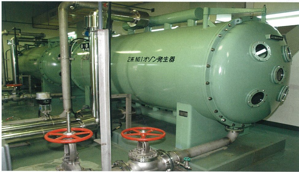
Advanced Water Treatment Facilities
